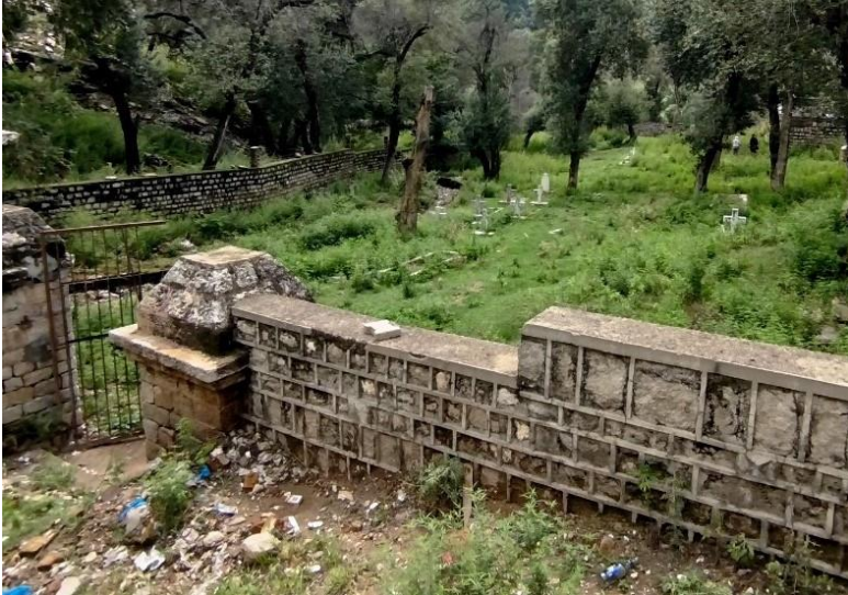
Malakand Cemetery, Pakistan, before work began Courtesy of Major General (Retd) Syed Ali Hamid
